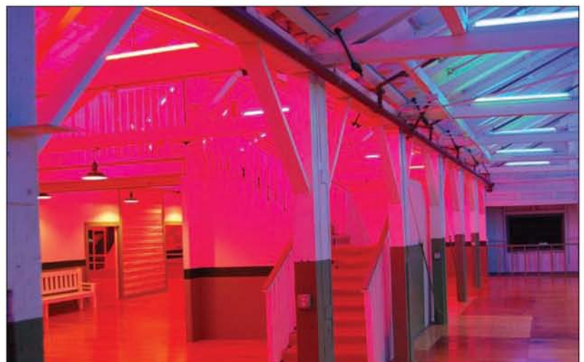
Gamtube™ color sleeves applied to fluorescent fixtures at McDermont Fruit Company Warehouse
